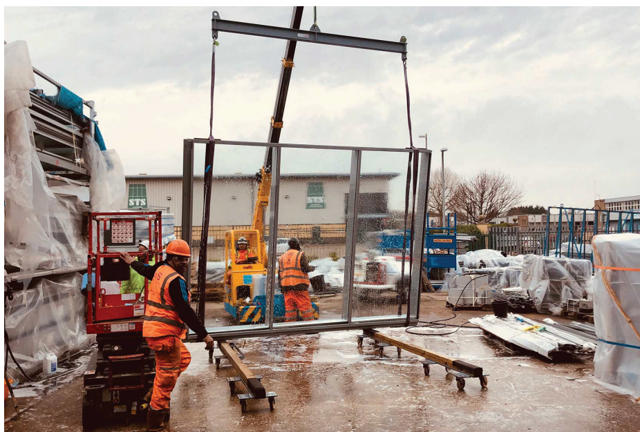
ONE TRITON SQUARE , in London, was originally designed by Arup in the 1990s, and the firm led its comprehensive retrofit more than two decades later (top). The curtain wall was disassembled and refurbished at a temporary fabrication site in the metropolitan region (above).
