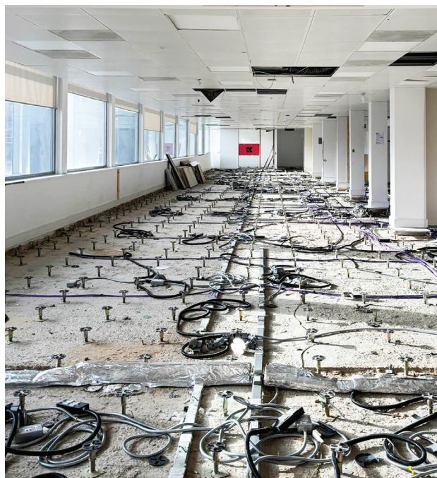
THE MARK has been soft-stripped of materials like raised access floors and carpet tiles (above).
