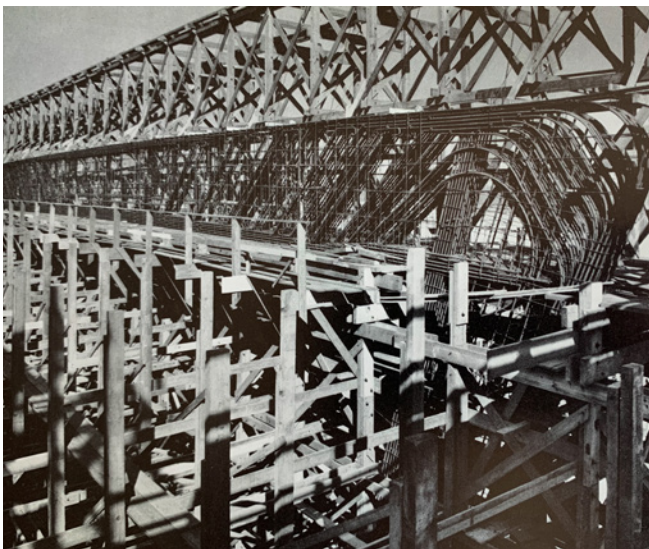
Figure 10. Detail of the upper frame reinforcement and formwork. Reidy and Portinho's shared love for exposed concrete was finally manifested in MAM, requiring precise framing and custom-cut 28 cm boards (typical was 31cm at the time) to achieve their desired surface finish. Image: (NPD/ FAU/UFRJ).
